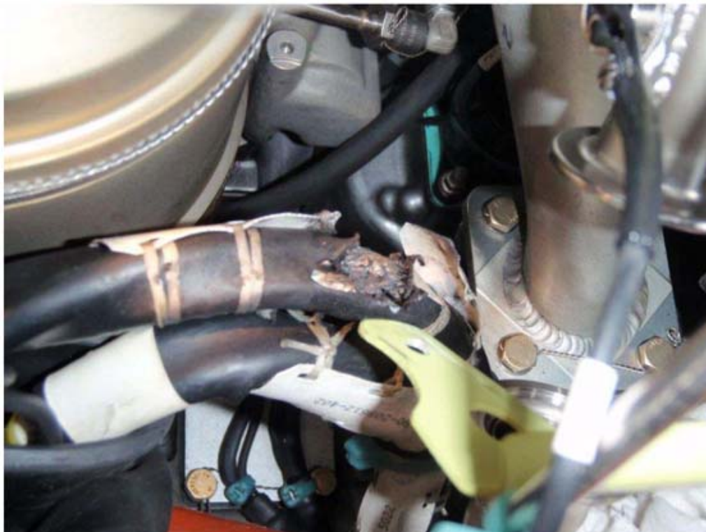
Fig. 210 - Damaged Power Cable
